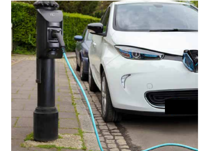
Figure 71: Example of on-street electric vehicle charging points.
