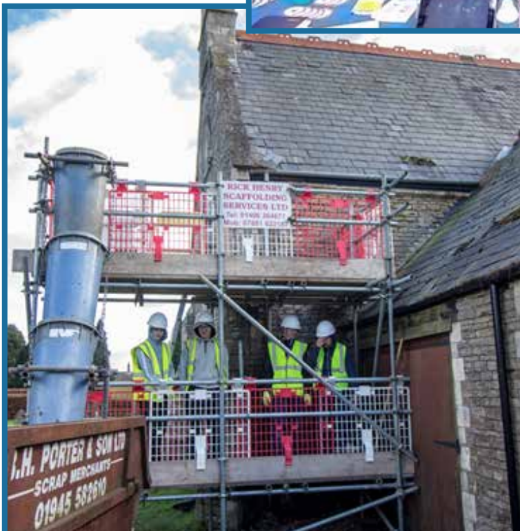
Bricklaying students from the College of West Anglia – one part of the Wisbech 2020 Vision project
