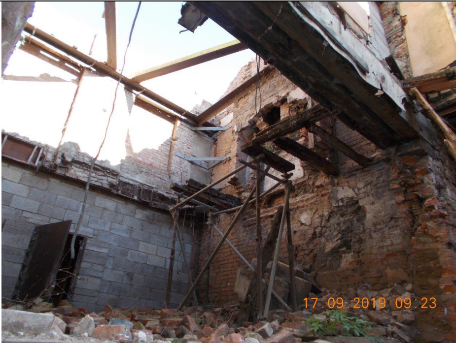
Area Requiring Urgent Works, 11-12 High Street, September 2019
