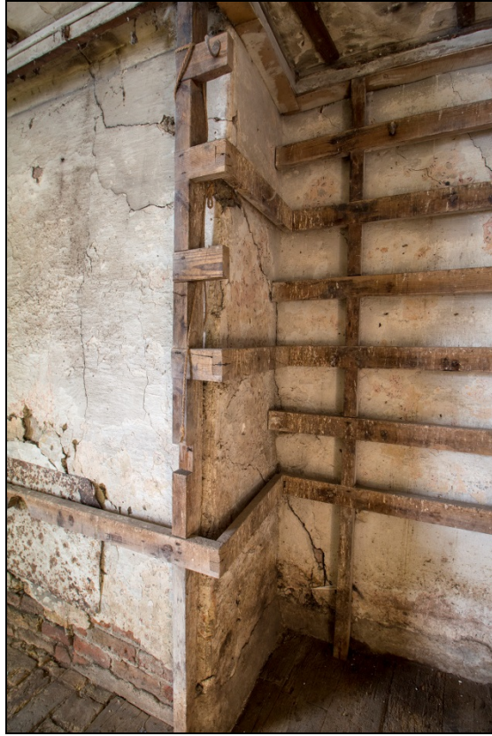
Detail of cracking in 2 nd floor room
