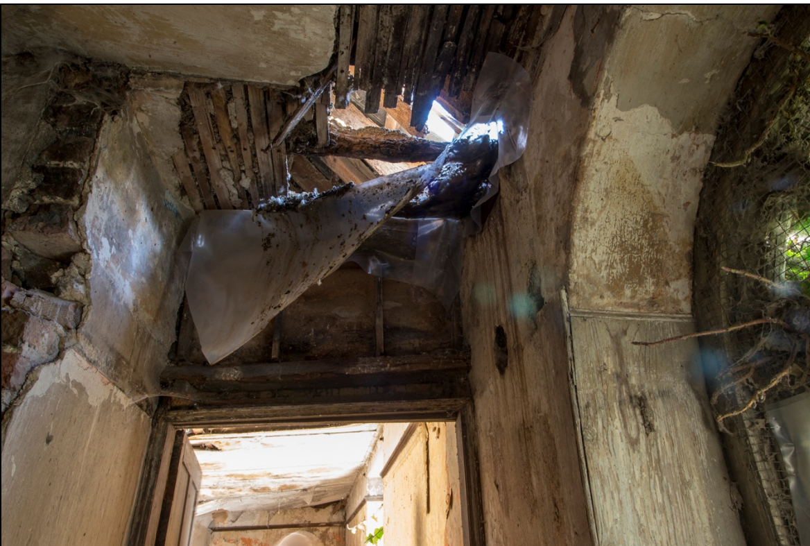
Damage to ceiling caused by missing roof covering
