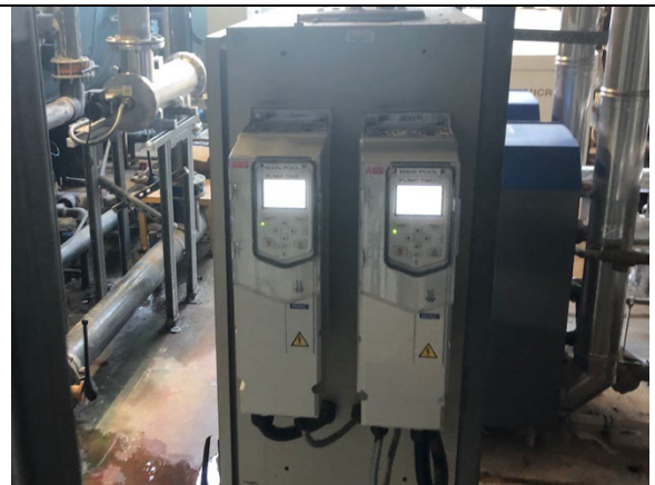
Circulating Pumps Inverter Control
