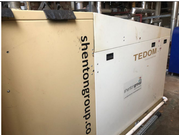
Non operational CHP
