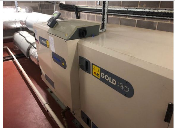
Heated Air System
