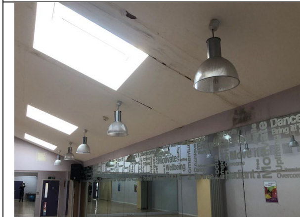
Gym lighting to be replaced
