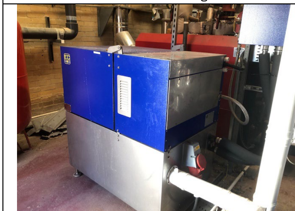
Non operational CHP
