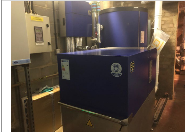
Non operational CHP
