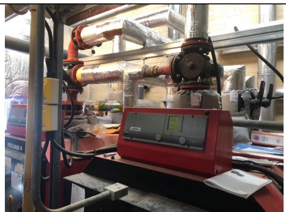
Boiler and uninsulated valve
